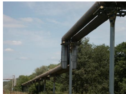
Figure 2. Double-circuit GIL in Częstochowa Steelworks
